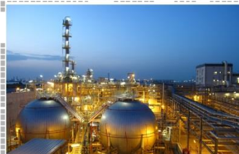
S-SBR plant (Singapore)
