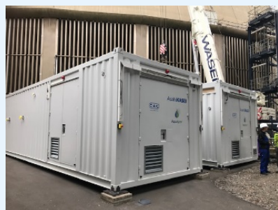
ALIGN-CCUS water electrolysis system (Niederaussem, Germany)
