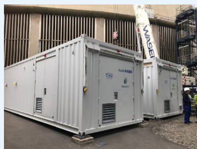
ALIGN-CCUS water electrolysis system (Niederaussem, Germany)
