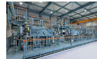
Alkaline water electrolysis pilot plant for hydrogen production at our Kawasaki Works
